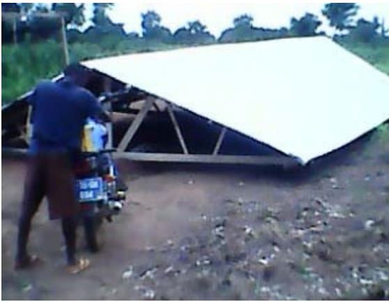
Kpandai Church building brought down by rain storm
